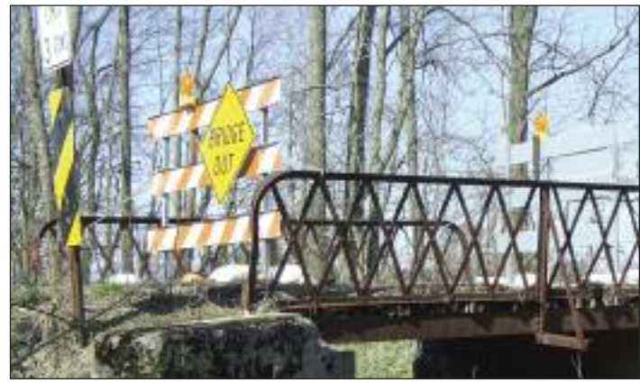
INQUIRER PHOTO/DEB PHILLIPS One Lane Bridge out on Twp. Road 51 east of Ohio 61 in Washington Township.
